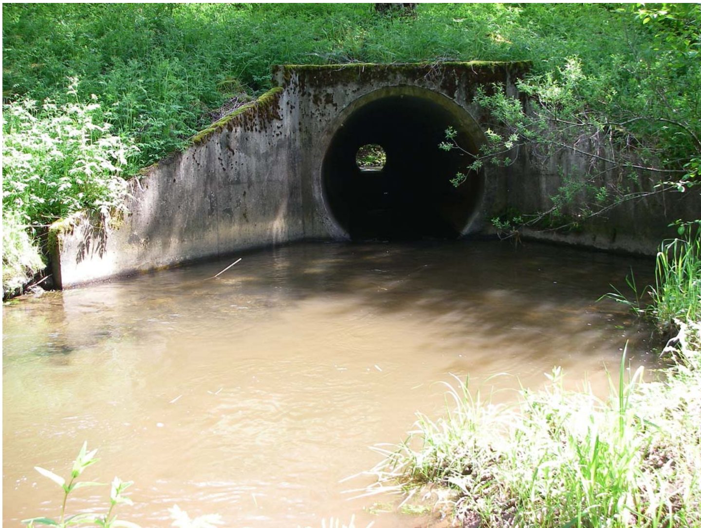
Photo 33. Under-sized HWY 26 culvert in Rock Cr Anchor Site 9. Compromising resource migration and delivery to lower mainstem Rock Cr.
