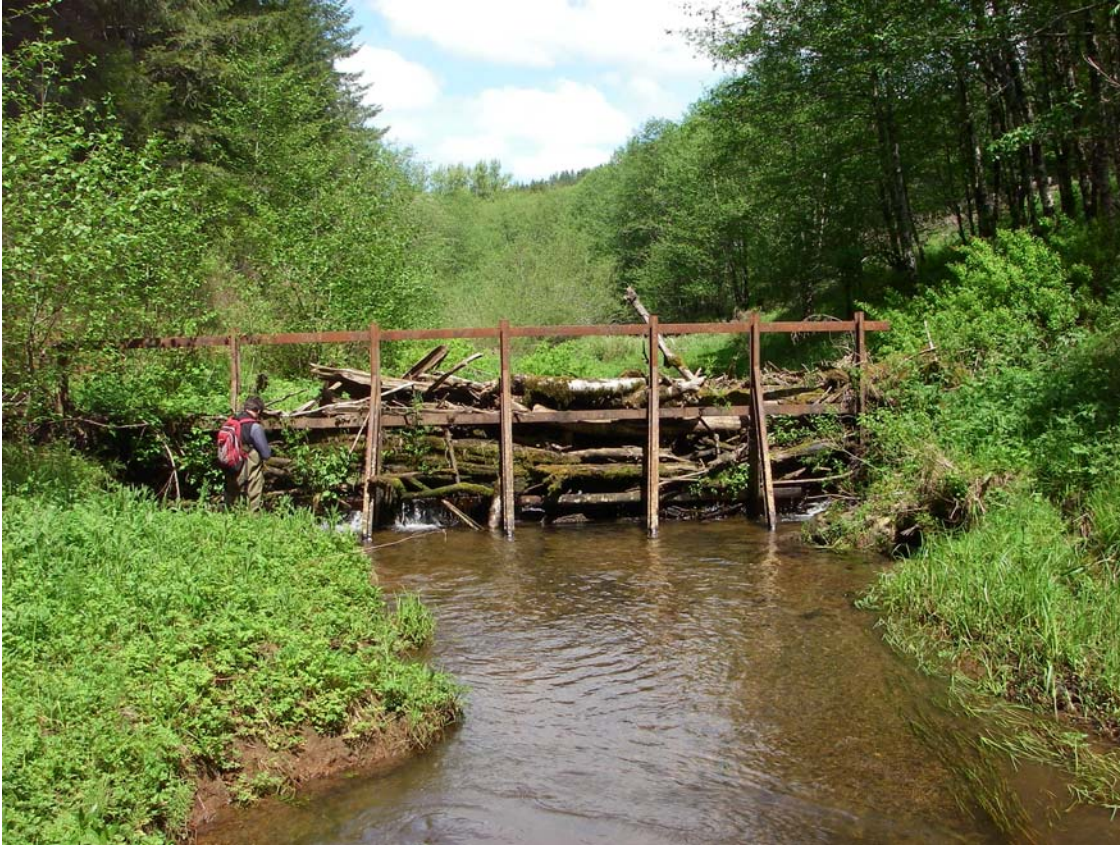
Photo 23. Un-maintained trash rack above HWY 26. Mainstem Rock.
